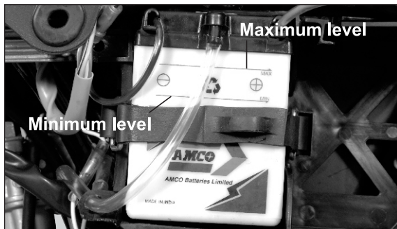
Battery electrolyte level
